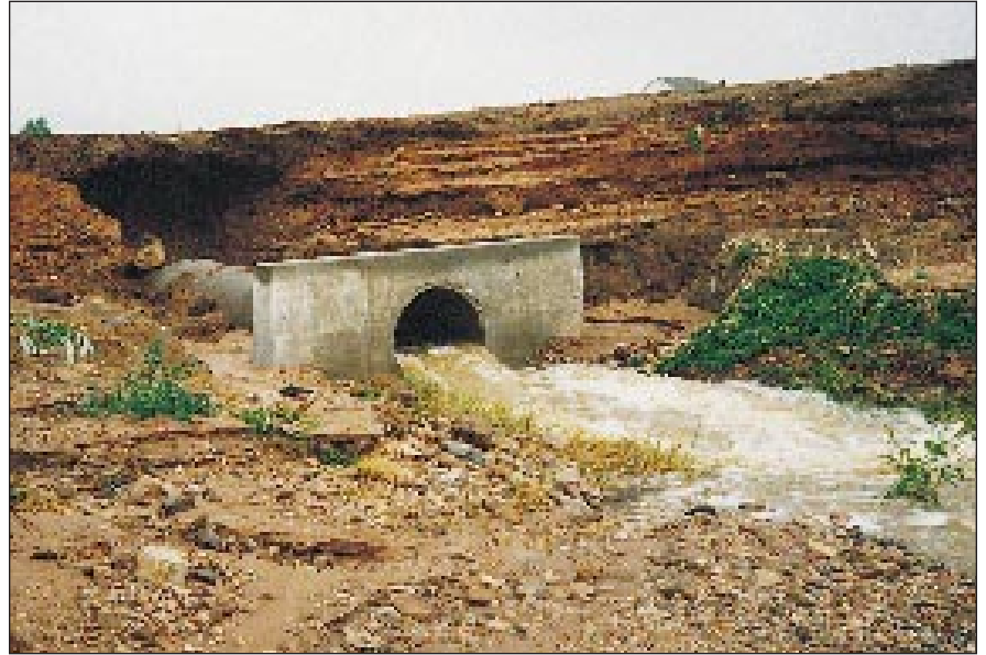
In the early morning hours of July 29, 1997, the devastation is obvious. Here, the east side of the Pleasant Valley and Lake Canal embankment has been scoured away by rushing overflow.
