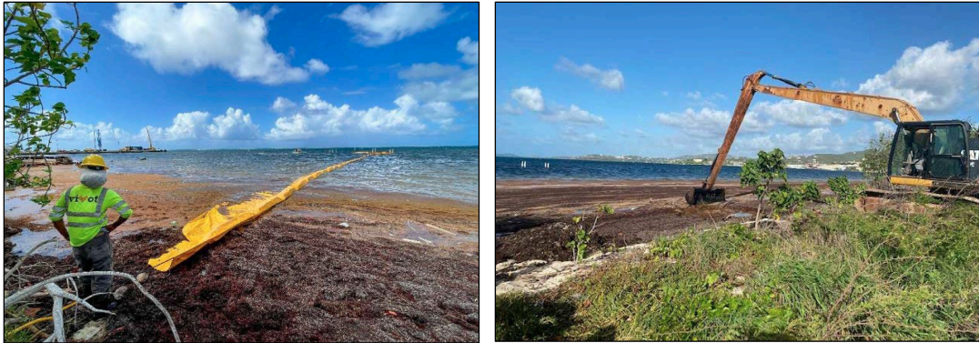
Figure 4-8. Response field operations. Boom maintenance using onshore personnel and small vessels, with Sargassum on the shoreline and in nearshore waters (left). Removing Sargassum from the shoreline using a long-reach tracked excavator (right). Source: FEMA.
