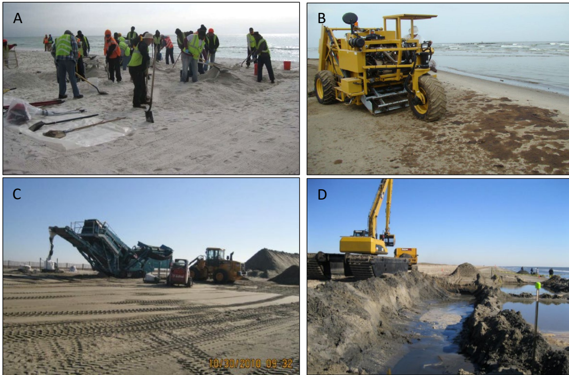
Figure 3-4. Examples of sand beach oil spill cleanup methods. (A) Manual oil removal using hand tools such as shovels, rakes, and small screens, which could also be used for oiled wrack. (B) Beach cleaning machine (Cherrington rake), which can be used to remove oil, such as tarballs, as well as oiled wrack. (C) Sifting of sediment piles created by mechanical removal to remove oiled material and separate it from clean or lightly oiled sediments. (D) Excavation of oil mats and debris, which could include buried oiled wrack deposits. Source: Michel et al. (2015).
