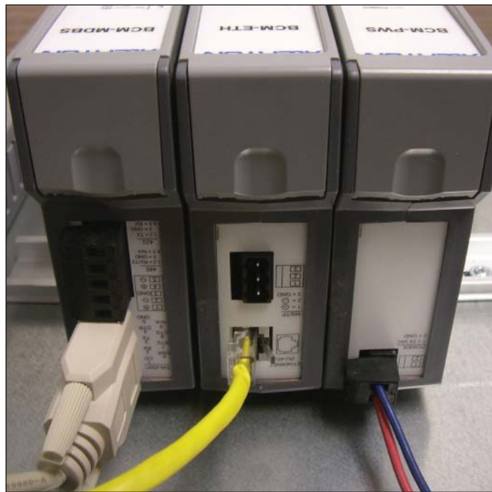
Figure 4: At bottom left, the SC110's DB9 female connector is attached to the BCM-MDBS. At center, a yellow Ethernet cable is connected to the Ethernet port on the BCM-ETH. The BCM-PWS connects to a 24 Vac source.
