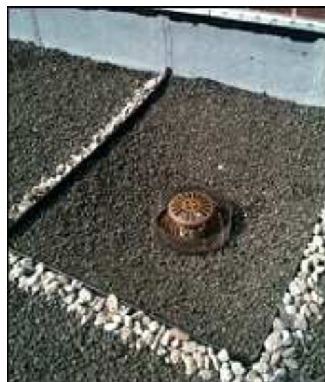
Figure 4: Weirs at the roof drain inlets create temporary ponding and more gradual release of water (NYC)
