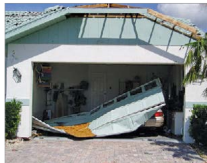
Figure 4-19. Because of their width, double-wide garage doors are more susceptible to wind damage than single doors. The wind can force it out of the roller track, especially if the track is lightweight or some of the anchor bolts are not in place. This occurs because the door fails under excessive wind pressure. Image courtesy of Florida Hurricane Depot.
