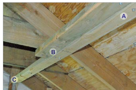
Figure 4-3. In this application of lateral bracing, the 2"x4"s are 18 inches from the ridge and connect to horizontal members that attach the opposing trusses. Not all roofs will have the horizontal members. The 2"x4"s are connected with two #14 3-inch screws (A) and overlap over two trusses (A and B). The end is connected to the gable end with an angle or L bracket (C). Image courtesy of Dennis Hwang.
