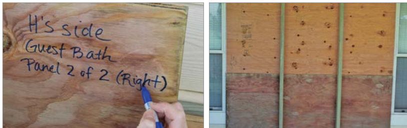
Figures 4-16 and 4-17. Not only is it necessary to install plywood opening covers correctly, it is also important to correctly label them and store them away from heat and humidity. Images courtesy of Dennis Hwang.
