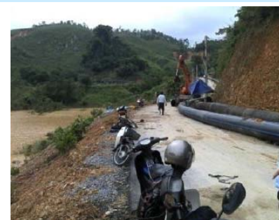
Burst water pipe
