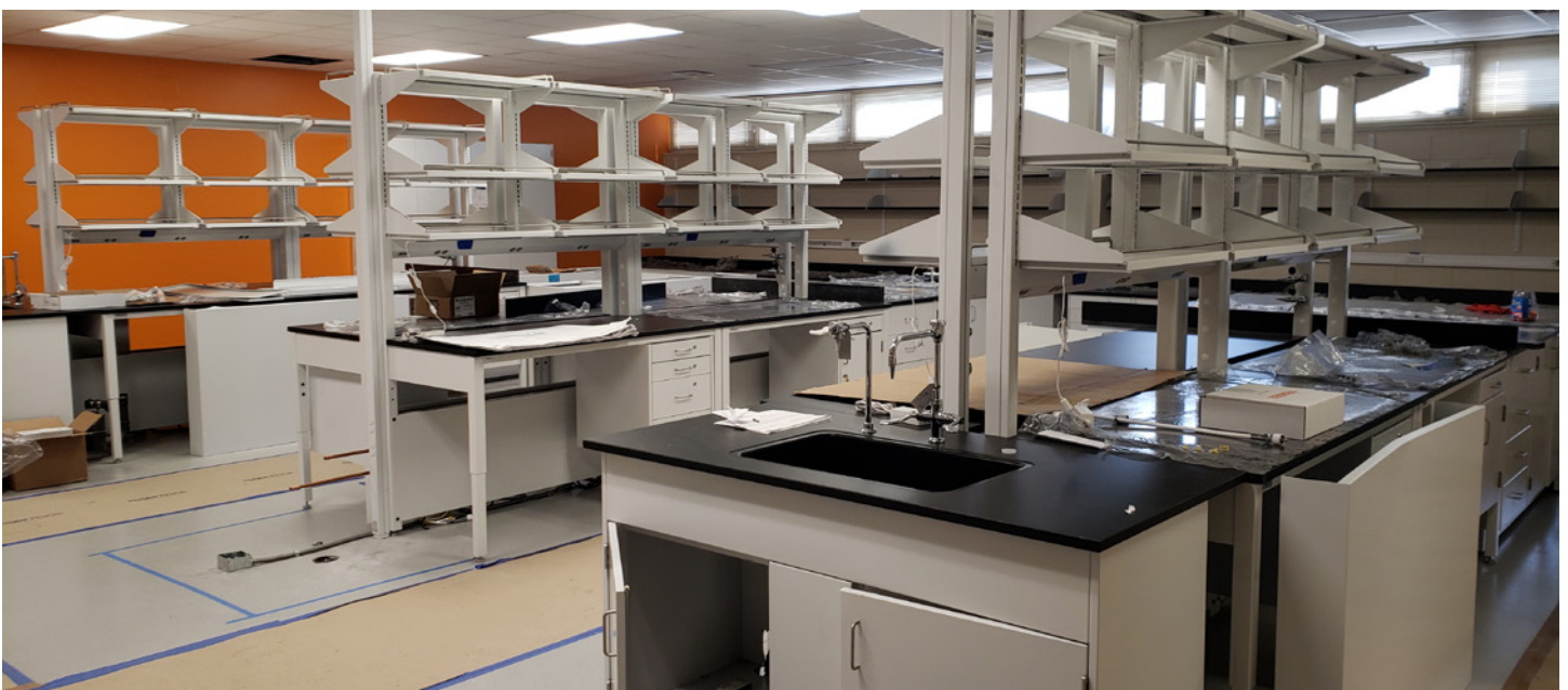
Pictured above are renovations taking place earlier in the year for the new Vector Borne Disease Laboratories. In addition to updating the aesthetics of the lab, several new pieces of equipment were purchased. Some of these equipment purchases are highlighted on pages 16-17 of the report.
