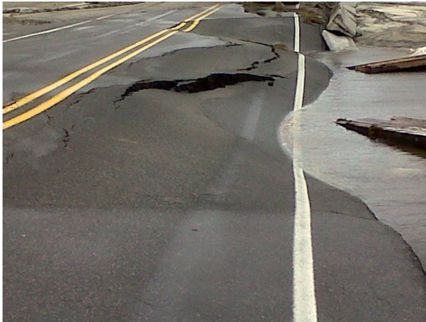
Temporary bridge and erosion of part of HWY 12 near Pea Island (right). Photo courtesy of NC DOT.
