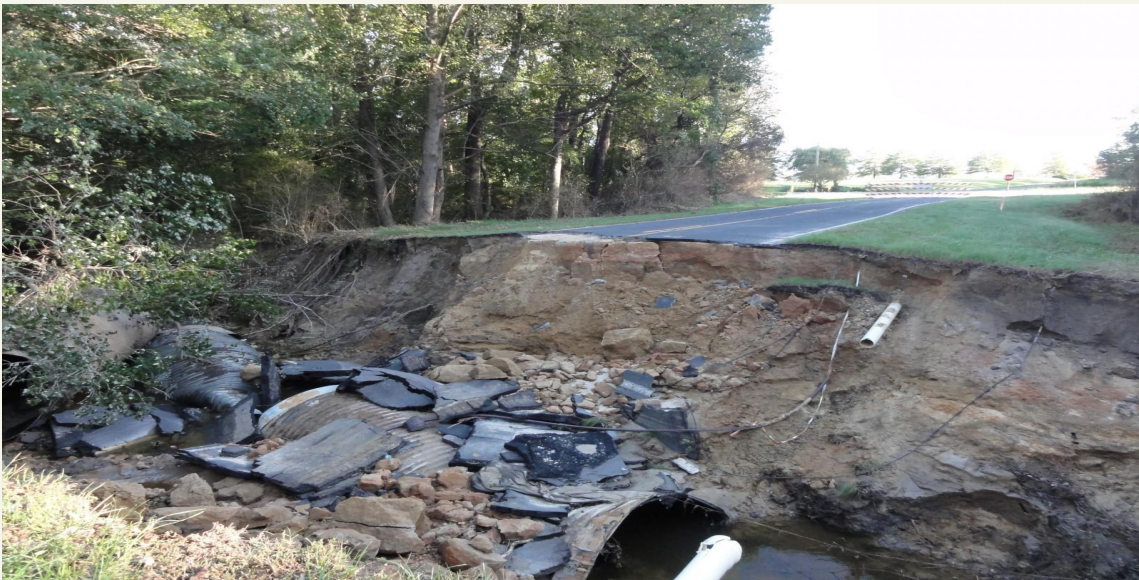
Washed out road in Greene County. This is why we urge folks when you see water covered roads to Turn Around, Don't Drown!
