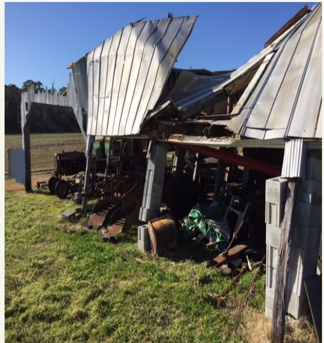
Damage from the Davis, NC tornado, February 16,
