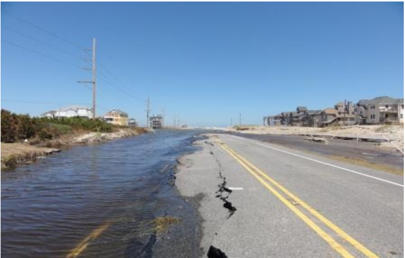
Hurricane Irene storm surge damage on Highway 12 along the Outer Banks
