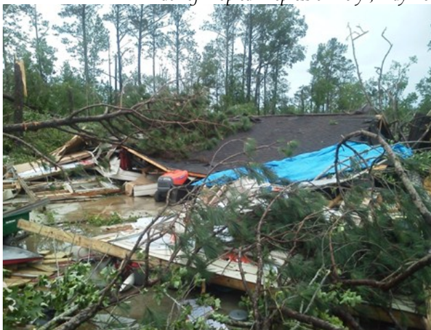
Tornado damage in Peletier, May 30, 2012
