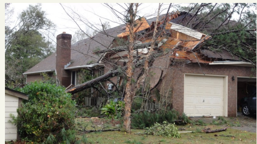
Damage in Morehead City
