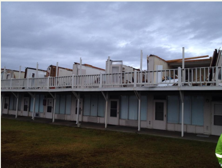
Damage to Ocean Sands Condominiums in Atlantic Beach
