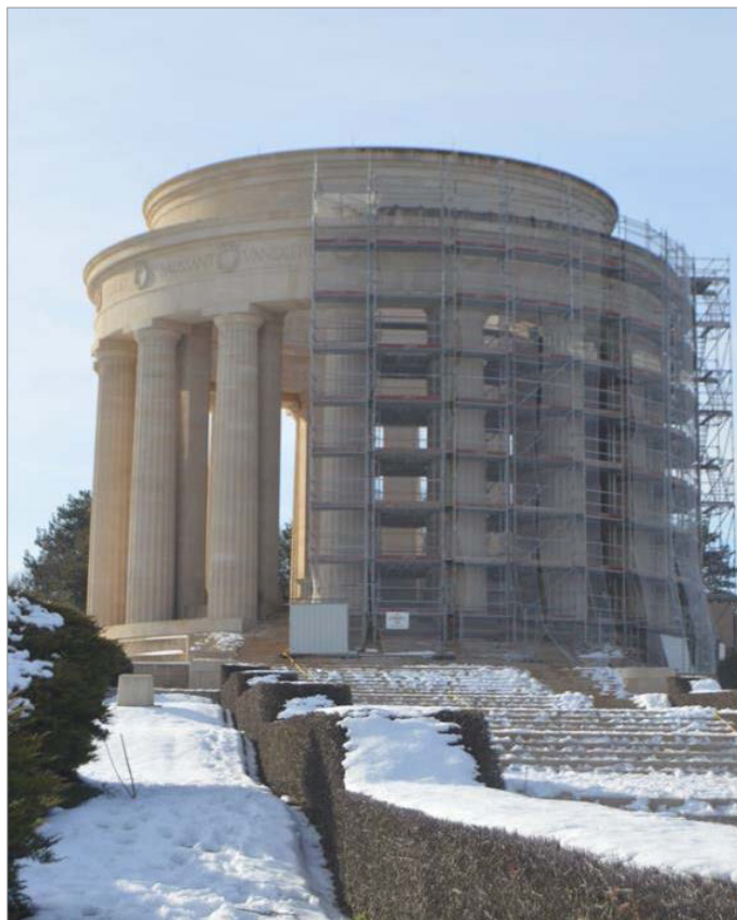
Scaffolding covers much of the Montsec Monument in France during a cleaning and restoration project
