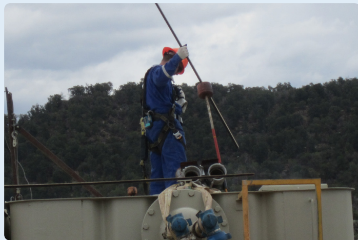
A worker manually gauges a flowback tank. The thief hatch is directly in front of his feet, and the gas and vapor released is invisible. Image: Max Kiefer, NIOSH.
