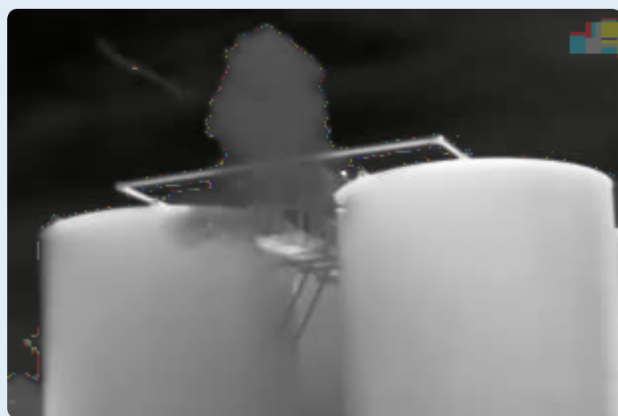
Forward-looking infrared (FLIR) photograph of the initial hydrocarbon plume after a thief hatch on a production tank battery is opened. The plume later expands to many times its initial size. Image: John Snawder, NIOSH.
