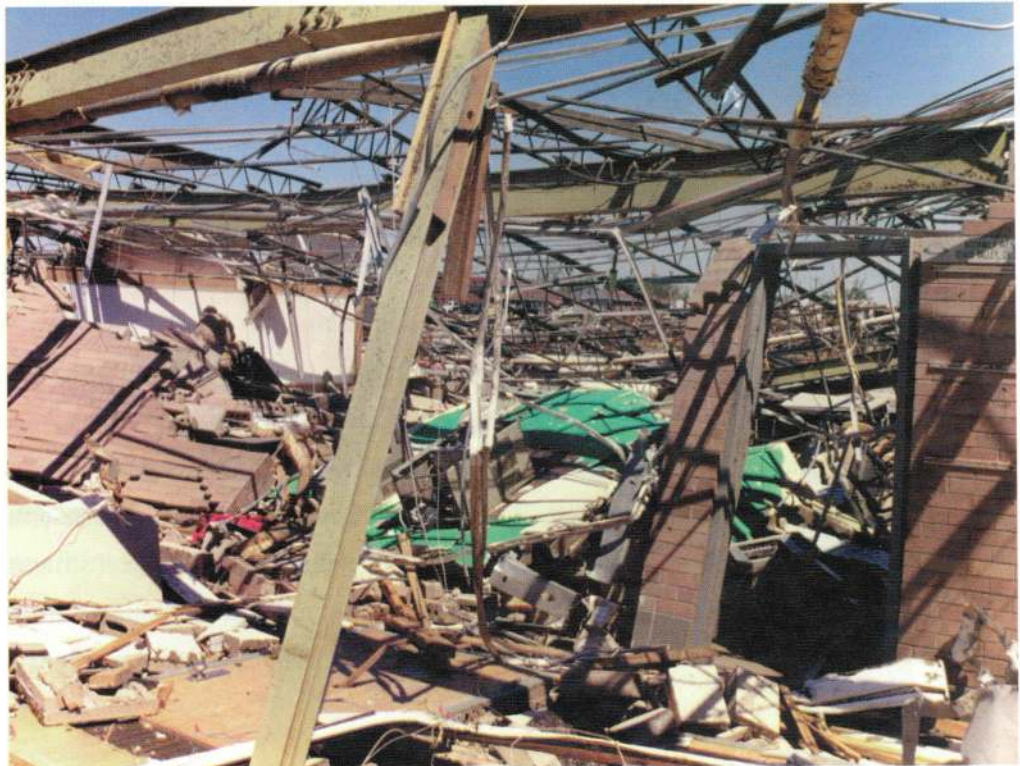
FIGURE 22. KELLY ELEMENTARY SCHOOL, MOORE, OK
