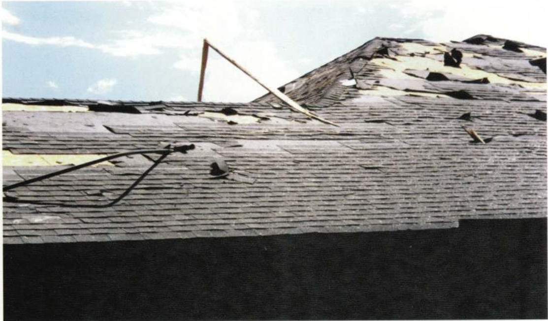
Figure 38. Steel Gas Pipe Projectile
