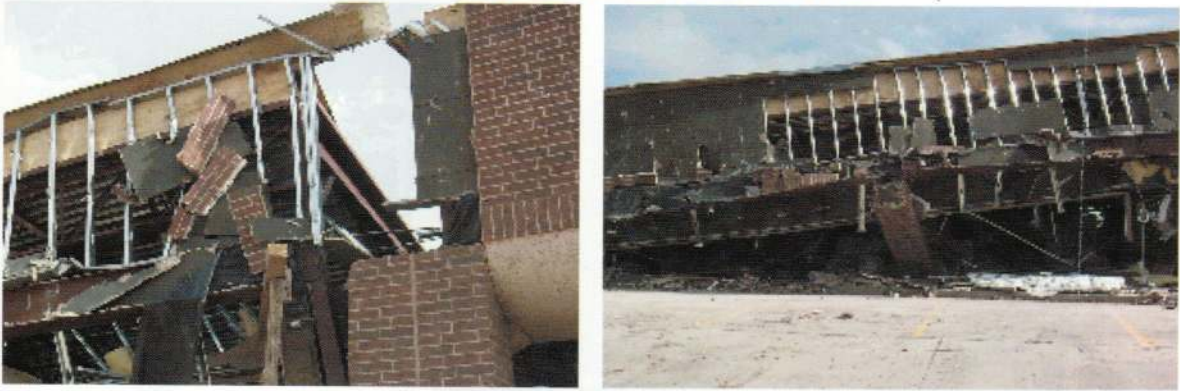
Disconnection of structural elements (left); collapse of the building addition (right).
