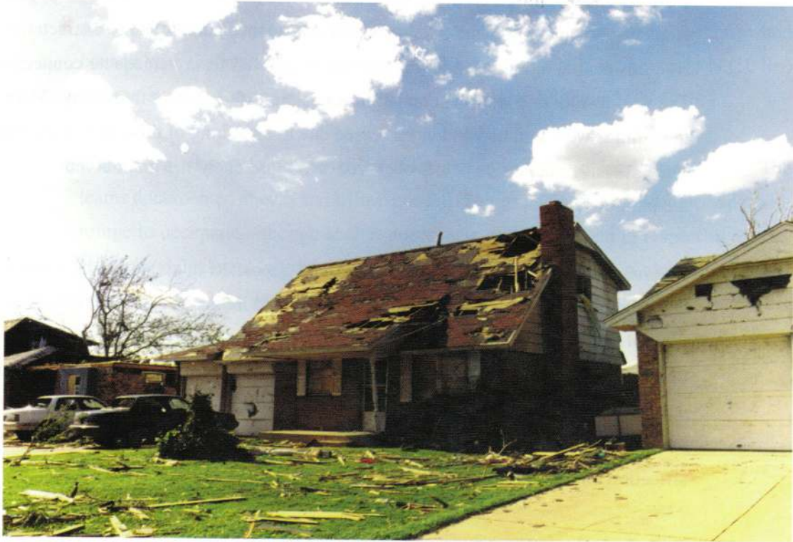
Figure 39. Homes Battered by Debris
