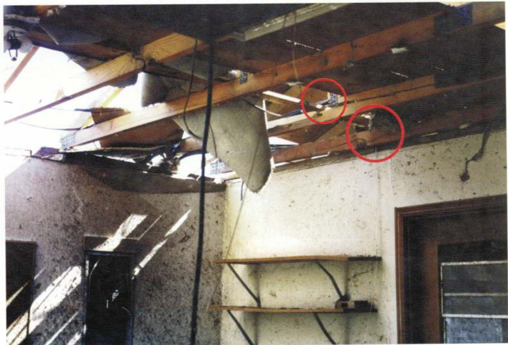
FIGURE 5. FAILURE AT KNOTS IN WOOD MEMBERS
