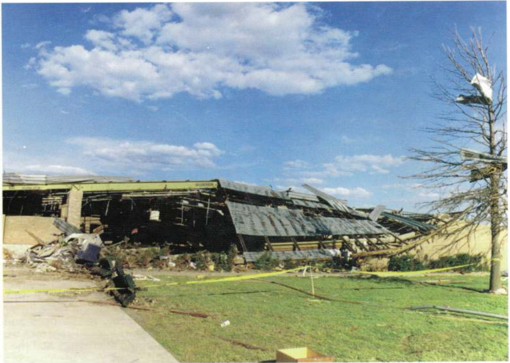
FIGURE 21. KELLY ELEMENTARY SCHOOL, MOORE, OK
