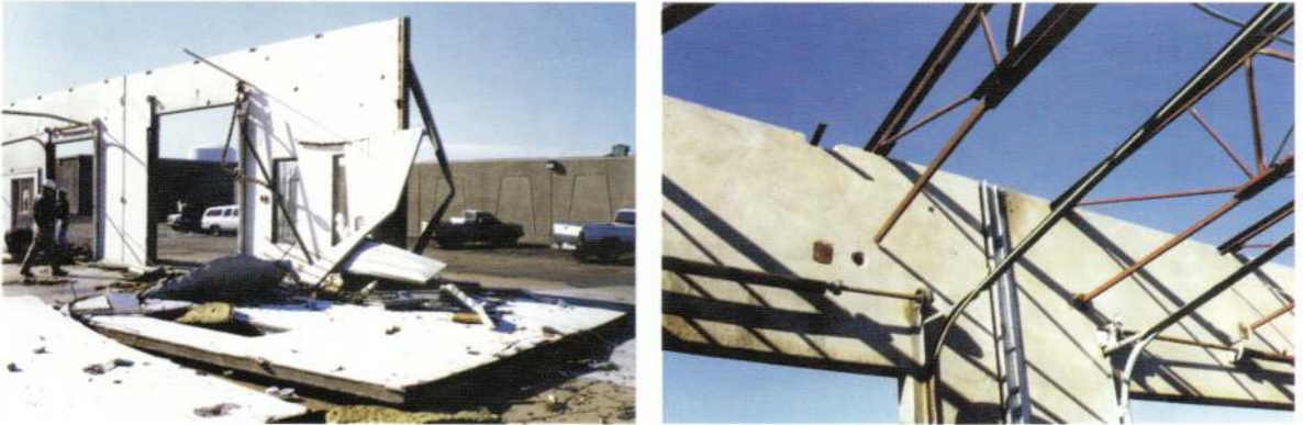
Lateral support failure of load bearing walls (left); failure of bottom bar joist chord connections (right).
