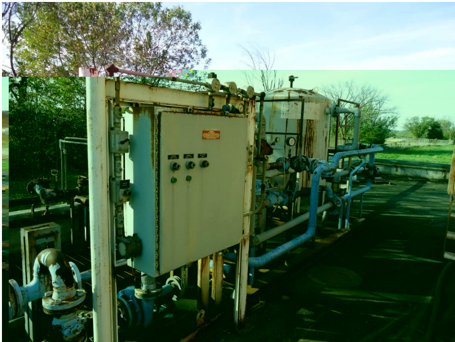
Water treatment system carbon bed
