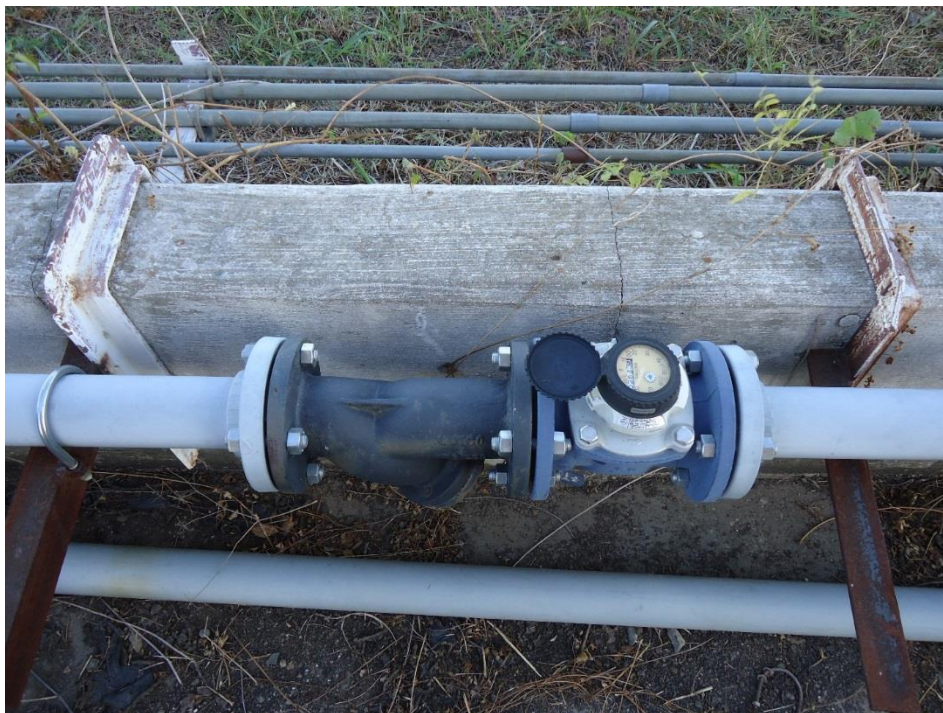
3-inch discharge pipe to POTW with totalizing meter
