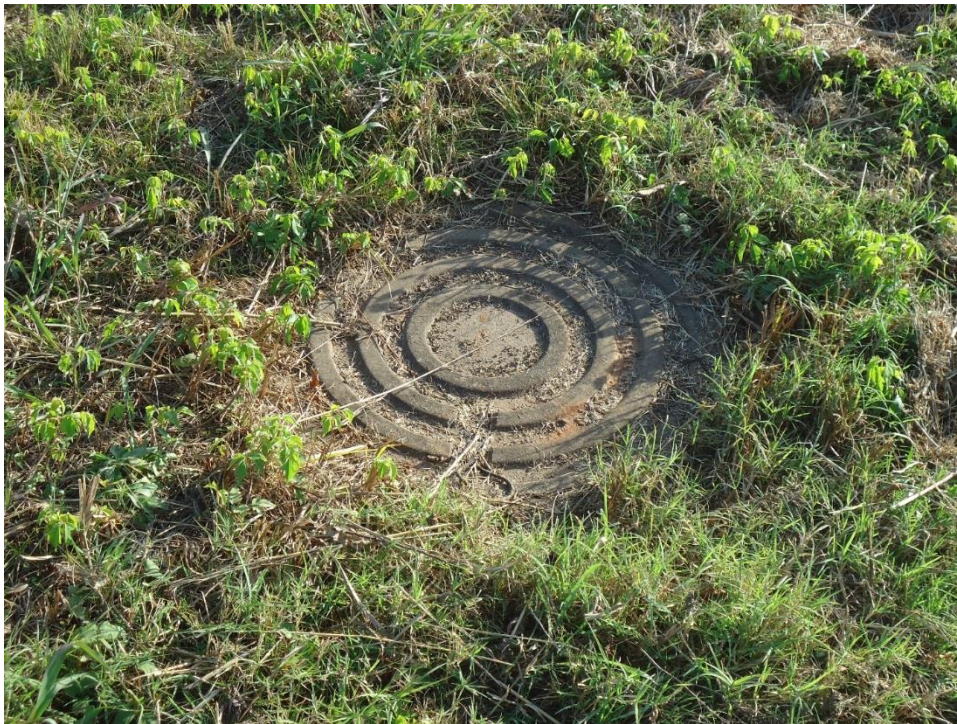
Sewer manway for sampling location for POTW discharges
