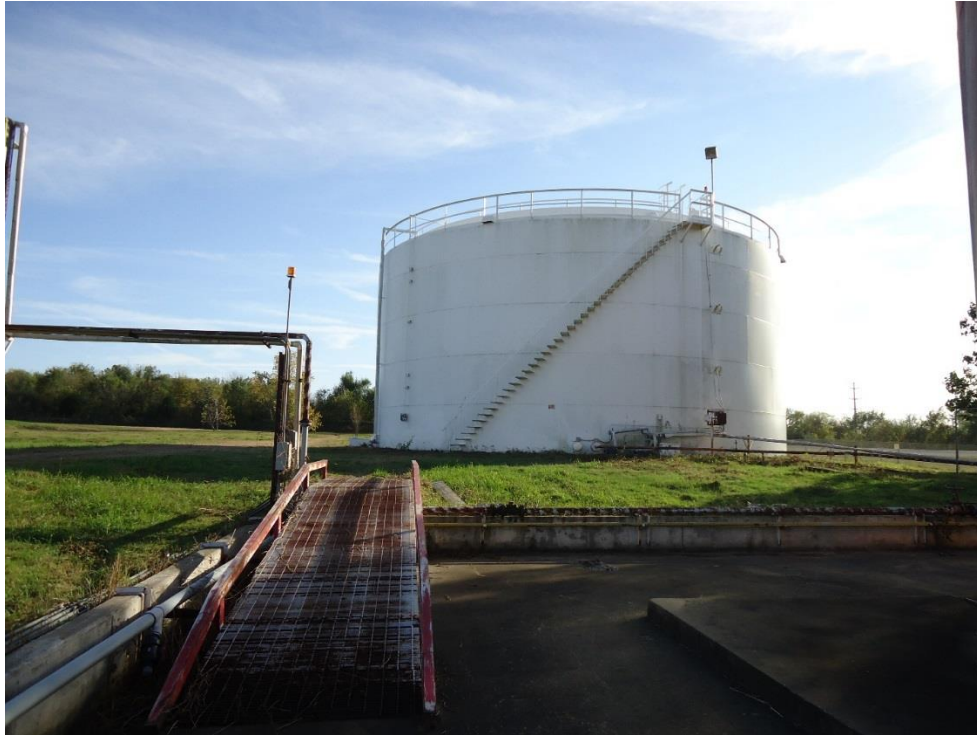
Groundwater collection tank V-69
