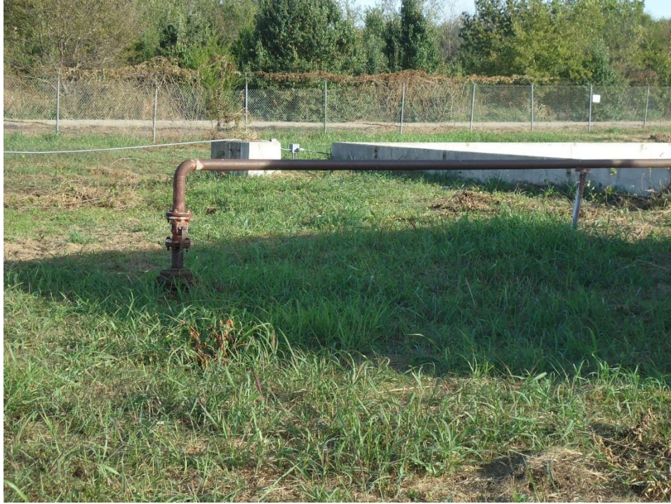
POTW discharge line entering underground sewer line
