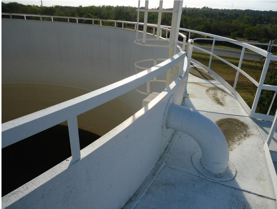
View of annulus walkway between the inner and outer tank (secondary containment)
