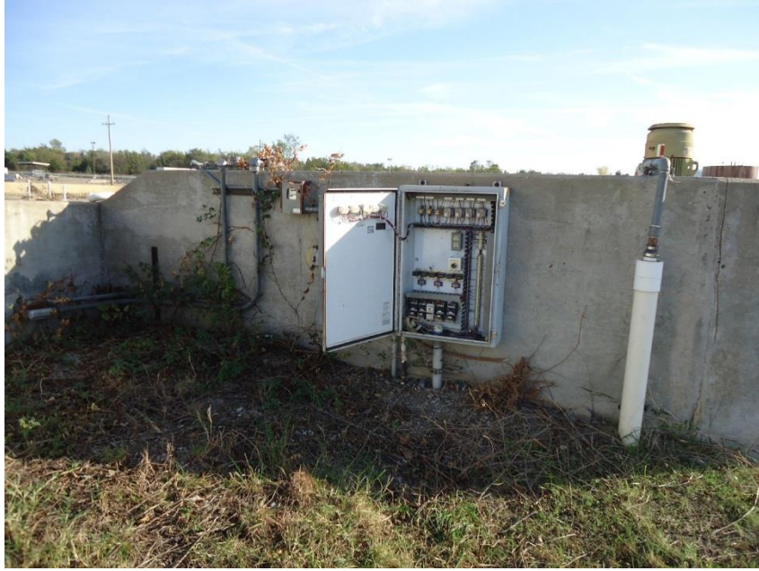
Groundwater collection system control panel
