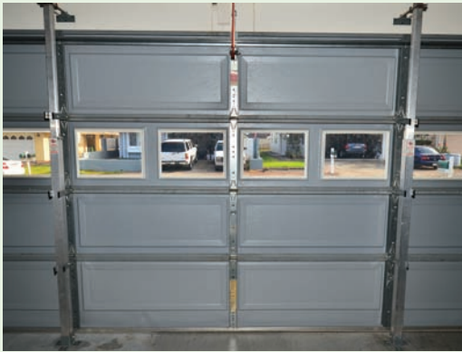
Figure 4-23. Vertical braces such as these can be deployed during high-wind events to strengthen the garage door. The braces are secured from the header over the garage door to the fasteners installed in the concrete floor. Deployment and breakdown are about 10 minutes each. The windows have been covered with a laminate film. Image courtesy of Dennis Hwang
