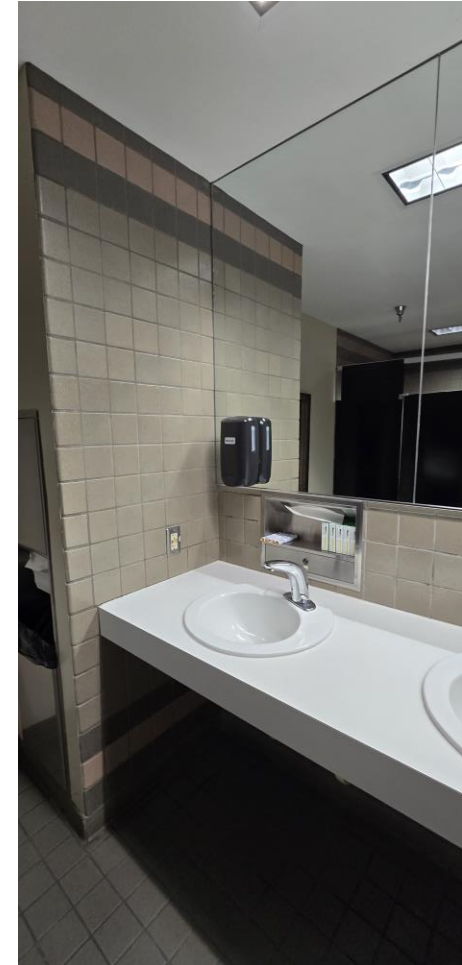
Automatic Soap Dispenser and Faucets
