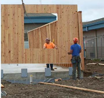
Cross laminated timber project building at Greywolf Elementary in the Sequim School District.
