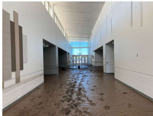
Figure: Mud and silt cover the floor of the Roswell Convention Center after flood waters receded. High water marks can be seen on the walls. Credit: Zachary Lujan
