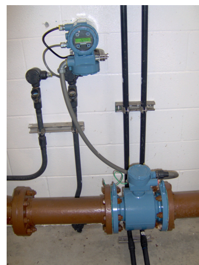
Installed Rosemount 8750WA Magnetic Flowmeter
