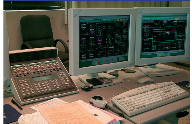
Dual CRT flat panel Ovation® Operator workstations are used to efficiently monitor and control the Sacramento Regional Wastewater Treatment plant processes.
