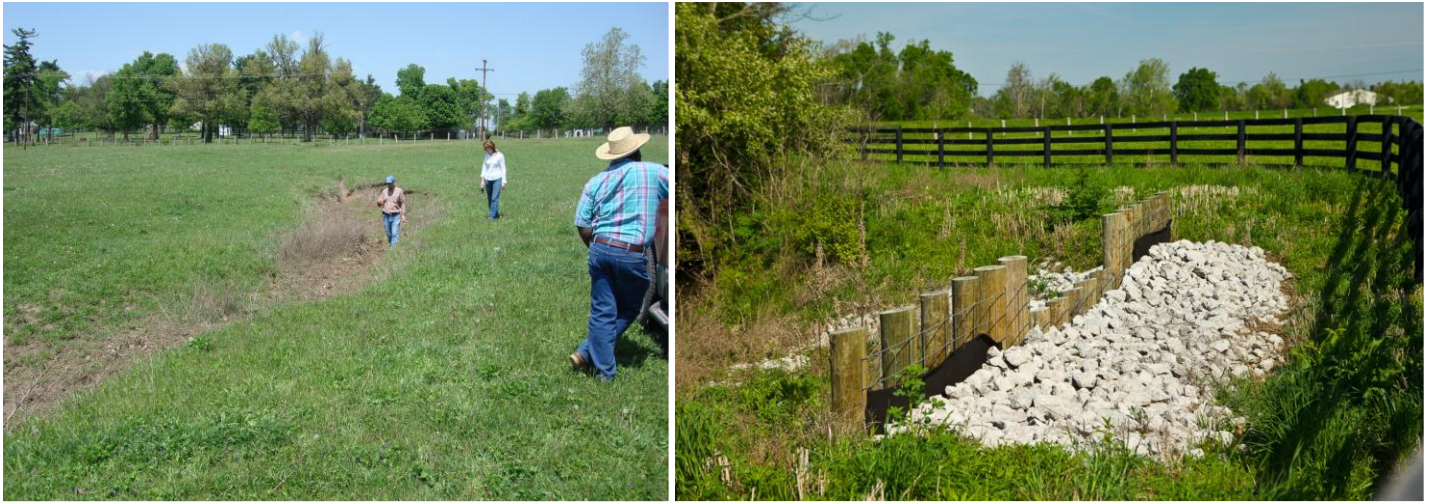
Figure 133. Eroded banks and washed out soil in a gully area near a Cane Run tributary; The grade stabilization structure prevents pollutants from entering the stream.
