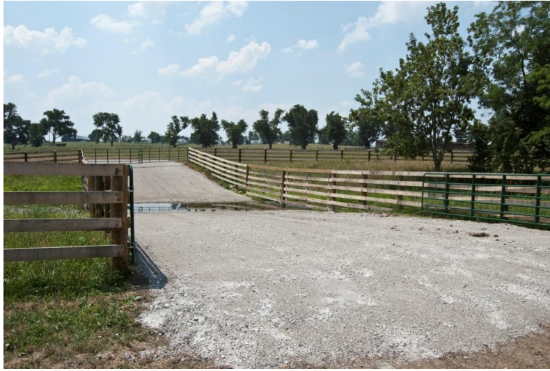
Figure 134. This hardened stream crossing prevents damage from livestock crossing
