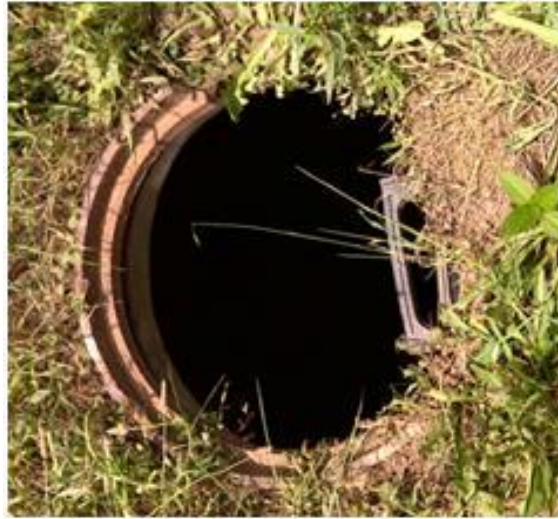
Figure 42. Manhole without cover
