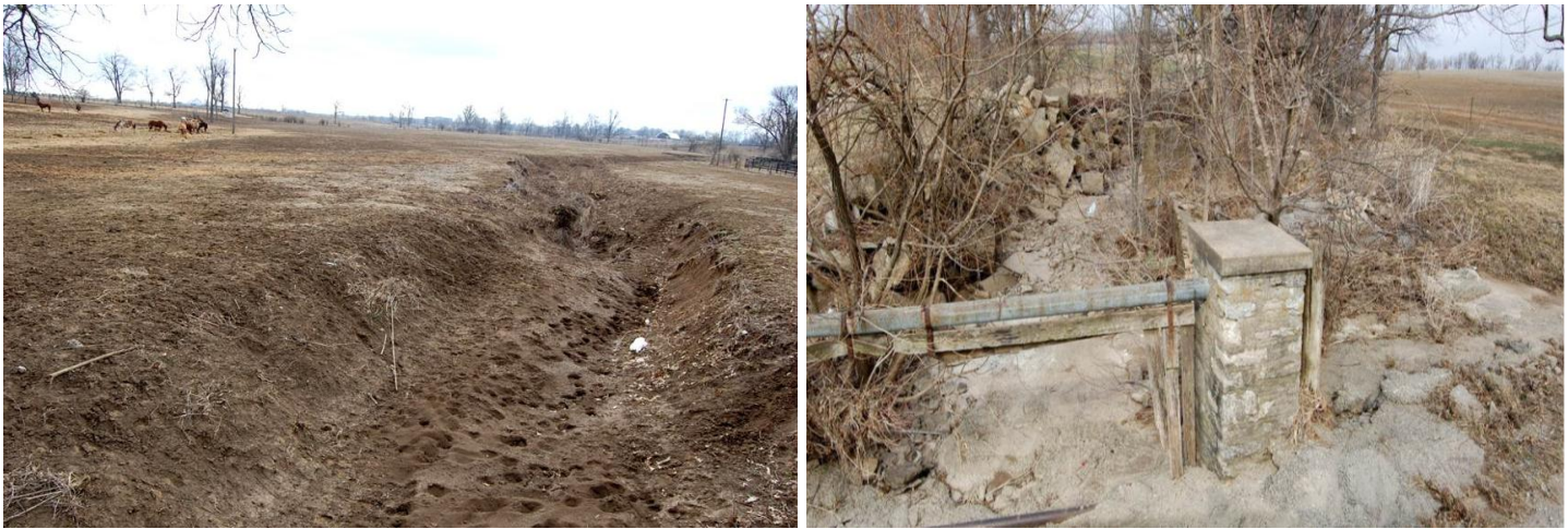
Figure 119. Erosion caused by a low water bridge; Concrete used to prevent erosion near low water bridge
