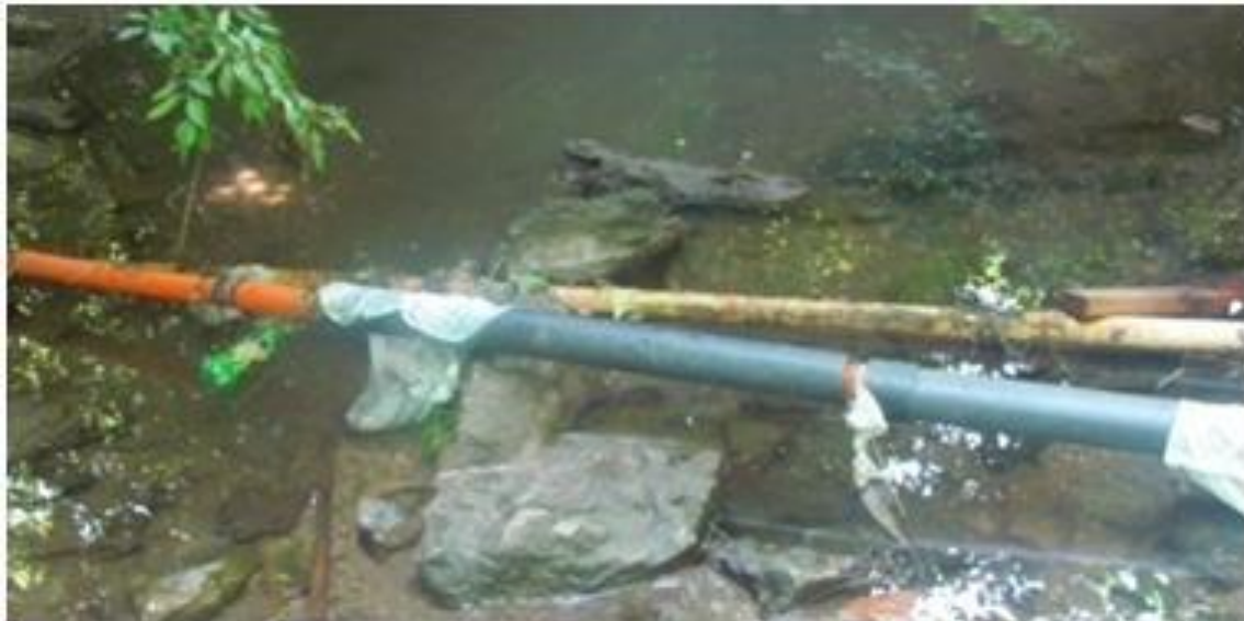
Figure 37. Utility line crossing stream
