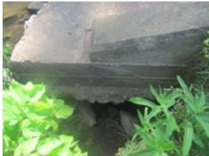
Figure 30. Bank eroded around endwall
