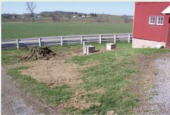
Milk house tank installed to collect waste and it will be field applied.
