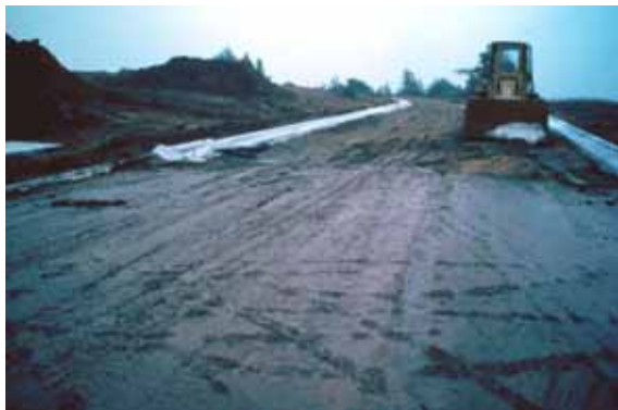
Construction site in early spring after snowmelt showing extensive sediment transport. SOURCE: Roger Bannerman.
