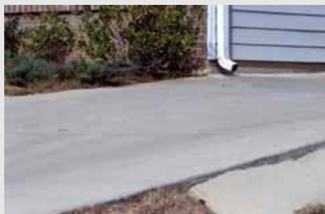
A directly connected roof drain
