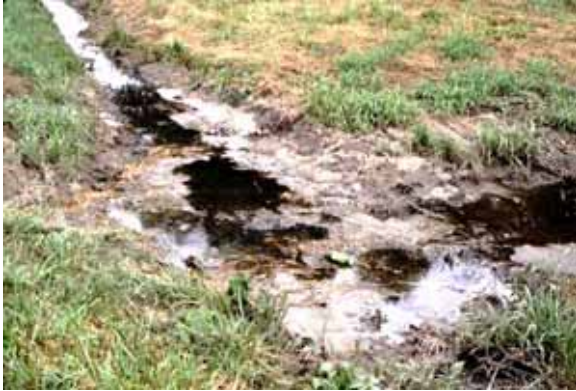
Failing sanitary sewer, causing upwelling of sewage through soil, and draining to gutter and then to storm drainage system.
