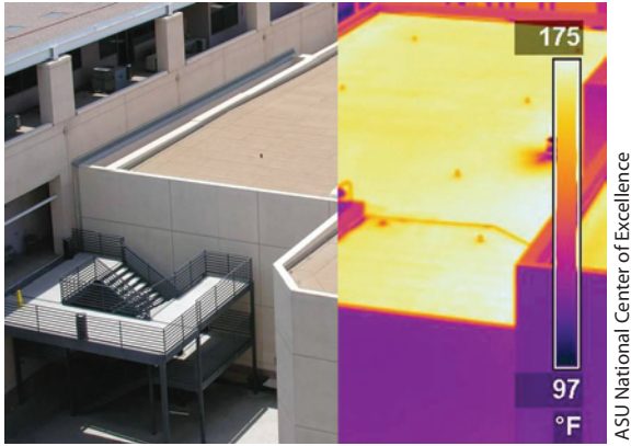
The left half of this traditional bitumen roof in Arizona is shown in visible wavelengths and the right in infrared. The roof's temperature reaches almost 175°F (80°C).
