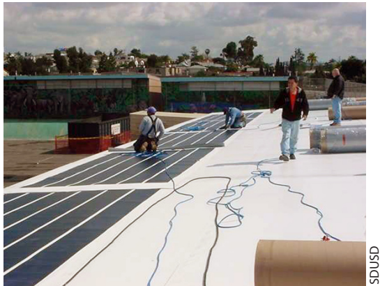
Figure 2: Cool Roofs with Solar Panels in San Diego
