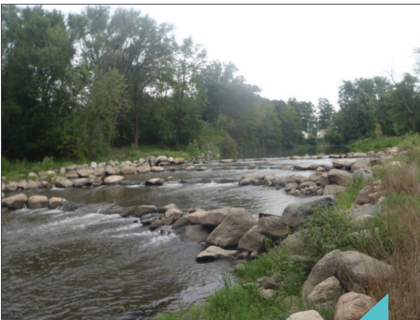
After the dam was removed from the Thornapple River in Nashville, Michigan, a four-tiered rock ramp was installed to improve stream conditions.
