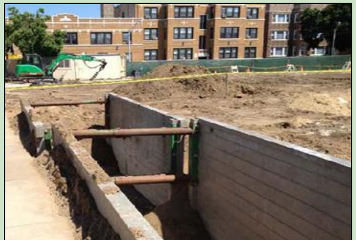
Mixing Trenches: At the Whitney Young Branch Library Brownfields Site, chemical oxidation reagents were mixed in three 16- by 16-foot trenches reinforced by steel. After mixing was complete, the steel was removed and reused onsite for purposes such as sidewalk shoring.
