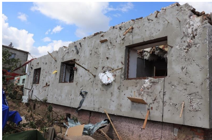
Figure 1-5. Debris impacts on the wall of a house in the tornado path.
