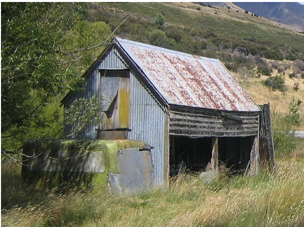
very weak frame with metal panels
