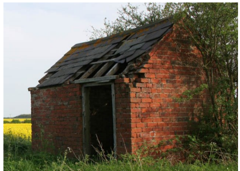
weakened brick wall structure
