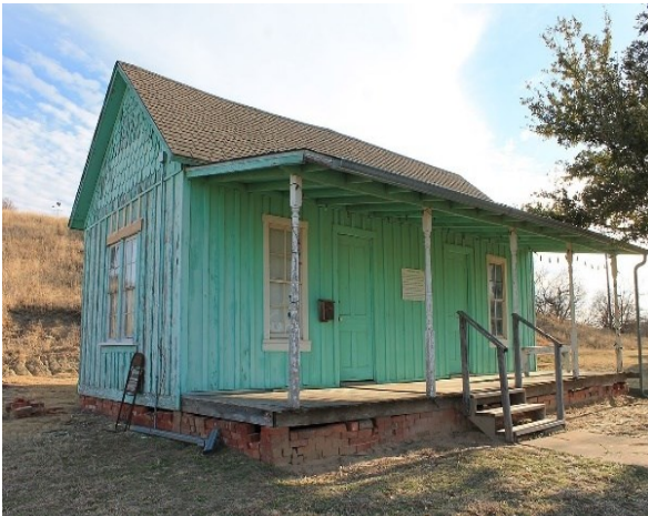
weak wooden frame with wooden panels
