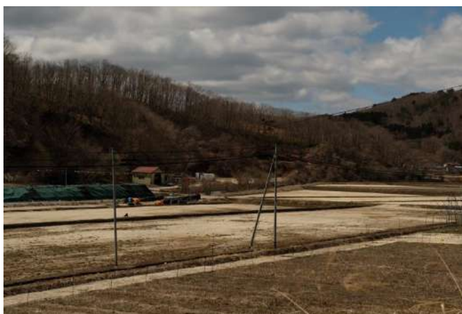
Photo 1. Large amount of non-contaminated soil (degraded granite soil taken from nearby mountains) dressed after decontaminating the paddy soil in Kawamata town, Fukushima (2016).
