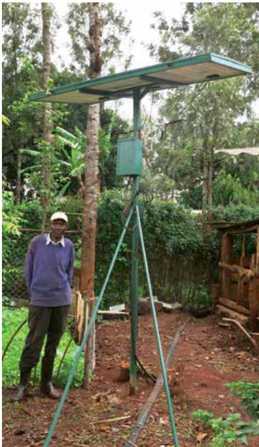
FIGURE 9 Elevated panels for a Solar Powered Irrigation System outside Nairobi, Kenya. Shading by trees is a problem
