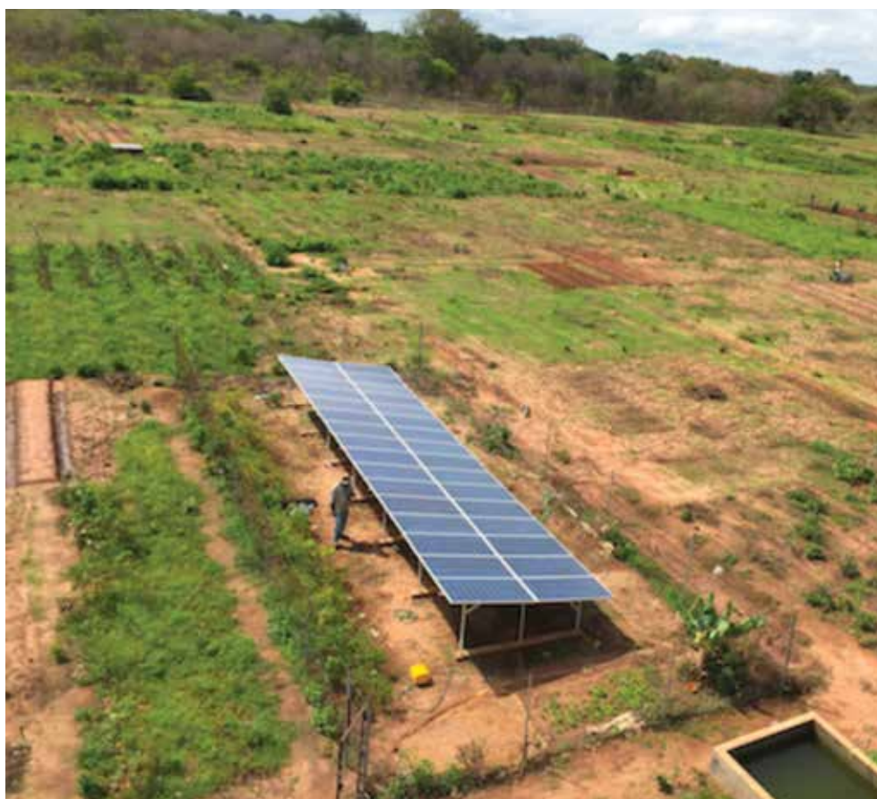
FIGURE 14 Solar Powered Irrigation System at Nuimi Lamin
