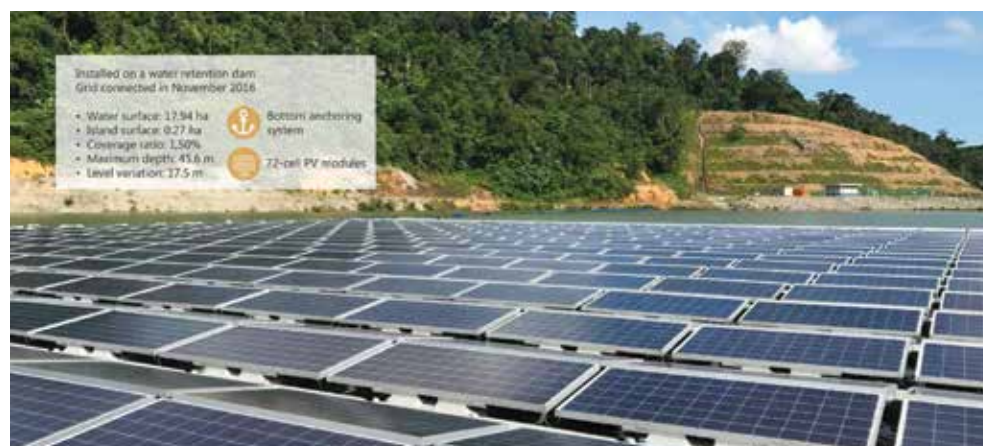
FIGURE 6 Floating solar system Ulu Sepri, Malaysia
