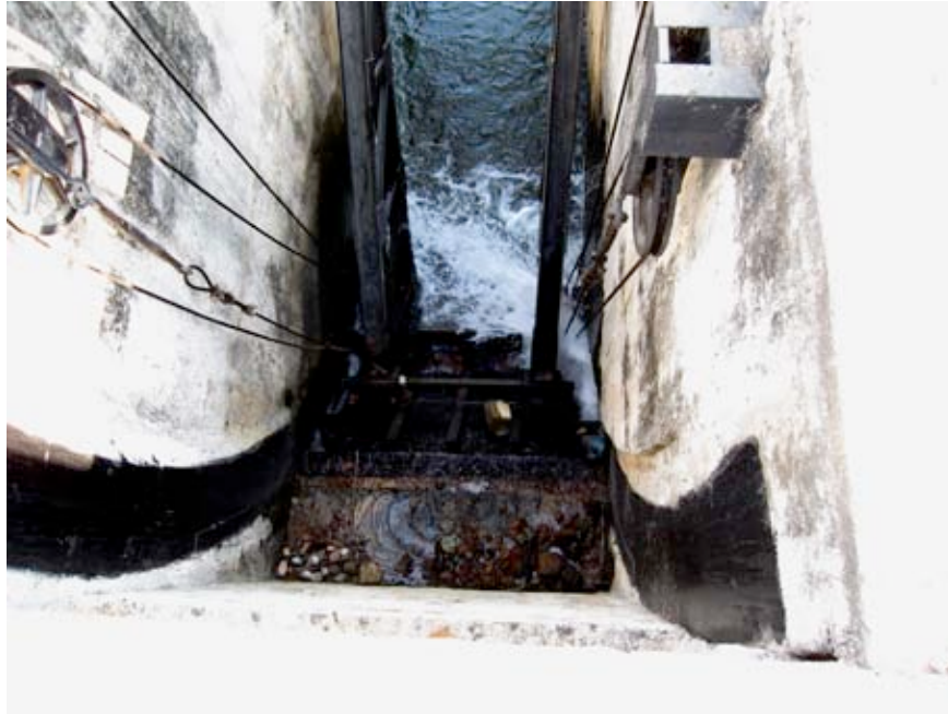
Plate 6. Servicing drainage escape ditch: non repaired leakage on an escape gate to served population along the drainage (Y Jonction Naryanpur canal)
