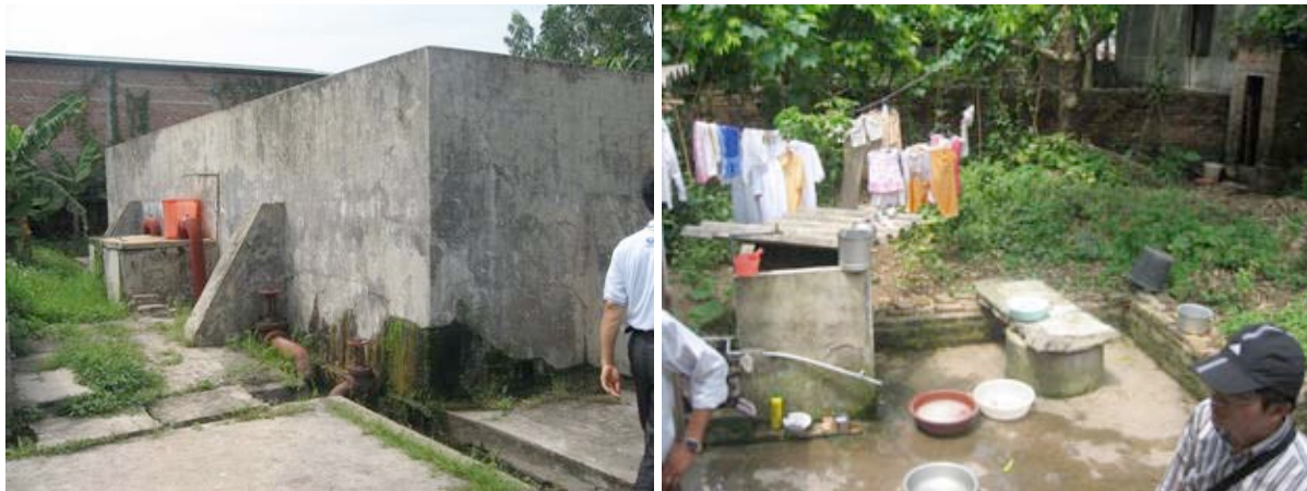
Plate 4: Water supply scheme to a town in Kim Dong district: left - water tank; right - tap in a house
