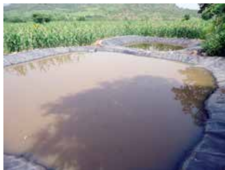
Figure 4: Rainwater harvesting ponds lined with geo-membrane
