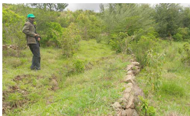
Rehabilitated catchment using excavated trench, stone bunding and grass reseeding at Miriam Monze watershed, Amhara Region
