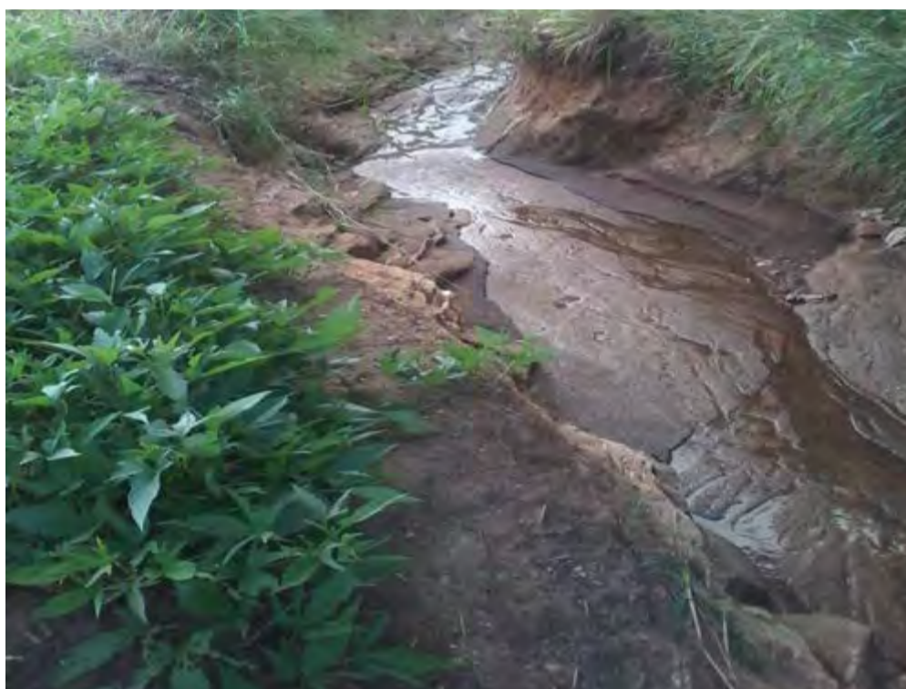
Riverbank erosion at Katunga
