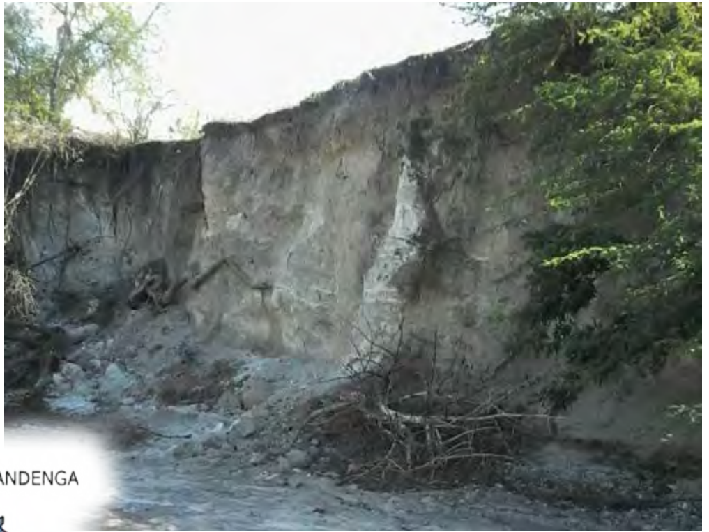
Riverbank erosion at Chibaya
