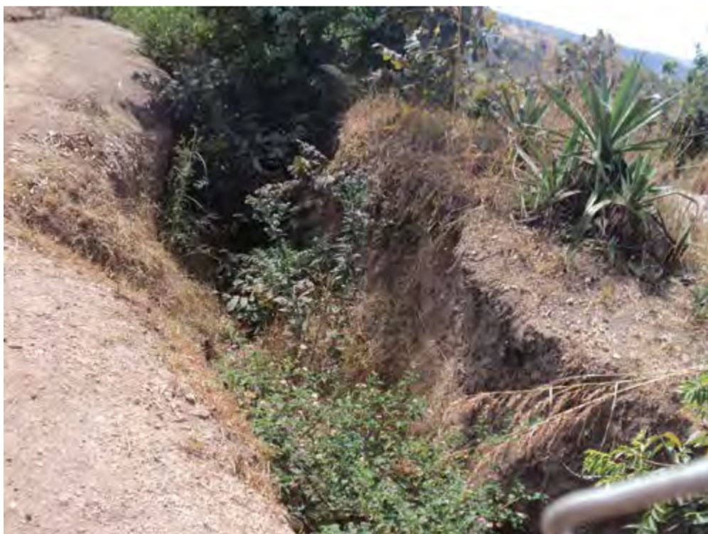
Gully erosion at Msakambewa
