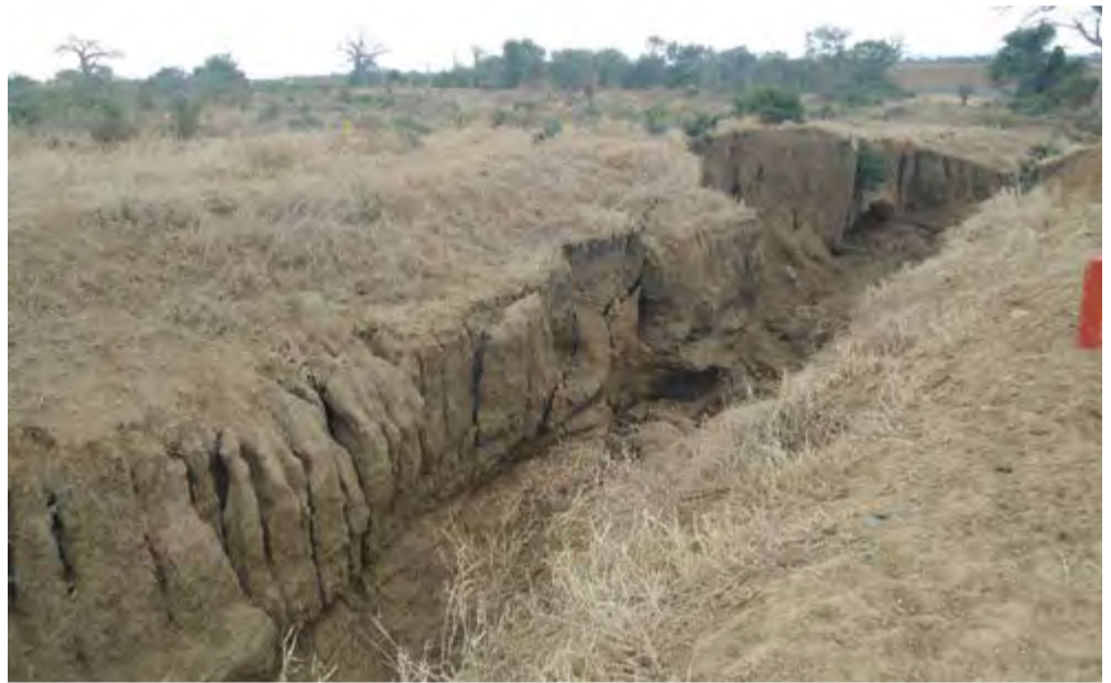
Gully erosion at Ndimbule village
