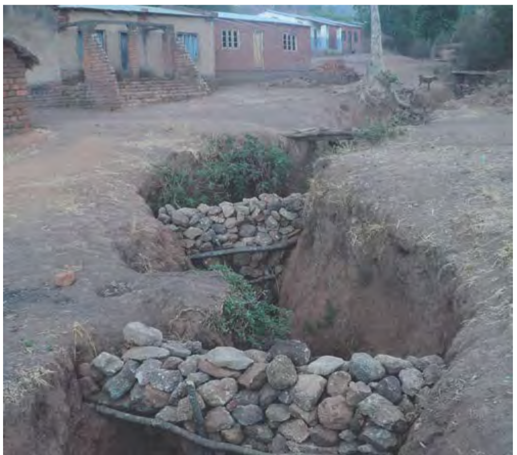
Sheet and gully erosion at Zidana village
