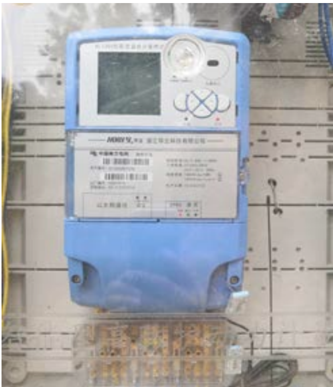
c. Electricity meter
