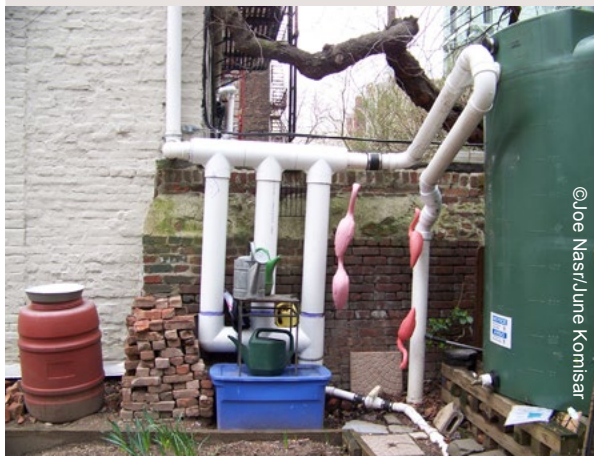
New York, USA. Rainwater collection system installed by GrowNYC in a community garden
