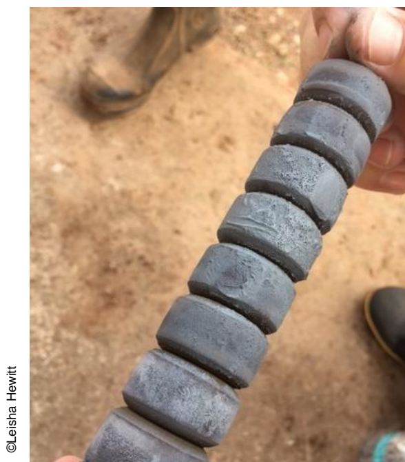
Figure 11. Build-up of residue around the recuperator sleeves
