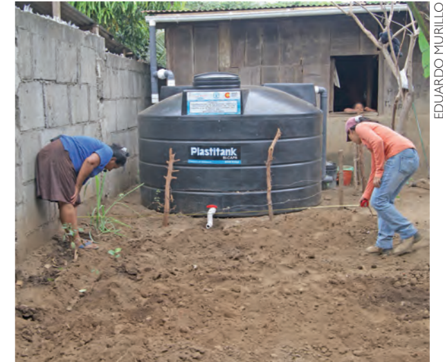
The project provided 430 rainwater harvesting systems, each linked to a 5 000 litre storage tank
