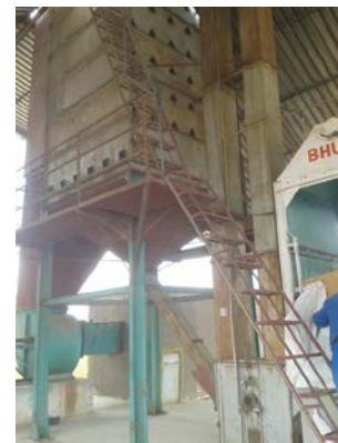
The construction seen underneath the dryer contains the rice-husk furnace.
