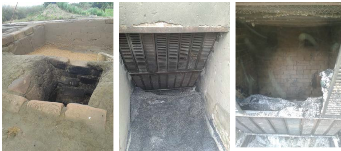
Entrance of the hopper on top: very little visible soot
