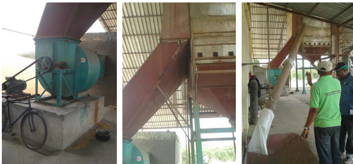
Figure13: Dryer hot air inlet and rice outlet
