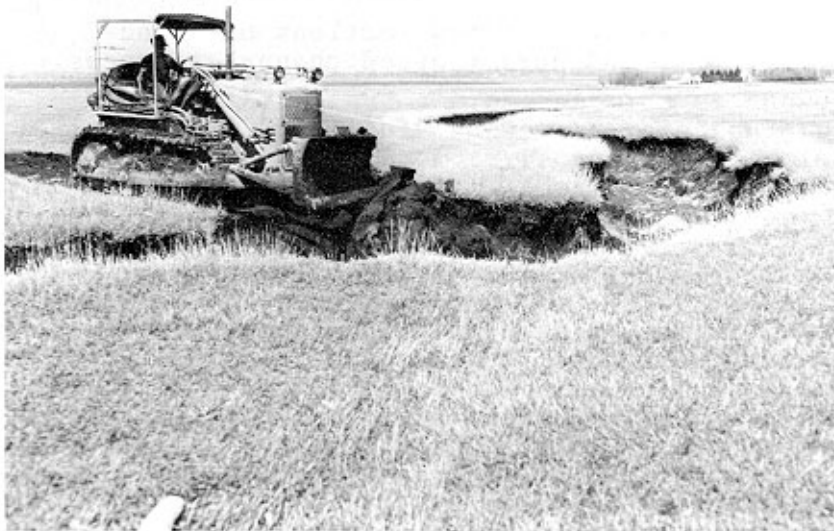
FIGURE 57. - Pushing soil into a gully prior to shaping and seeding for use as a grassed waterway. (Dakota, U.S.A. Photo courtesy of USDA Soil Conservation Service)
