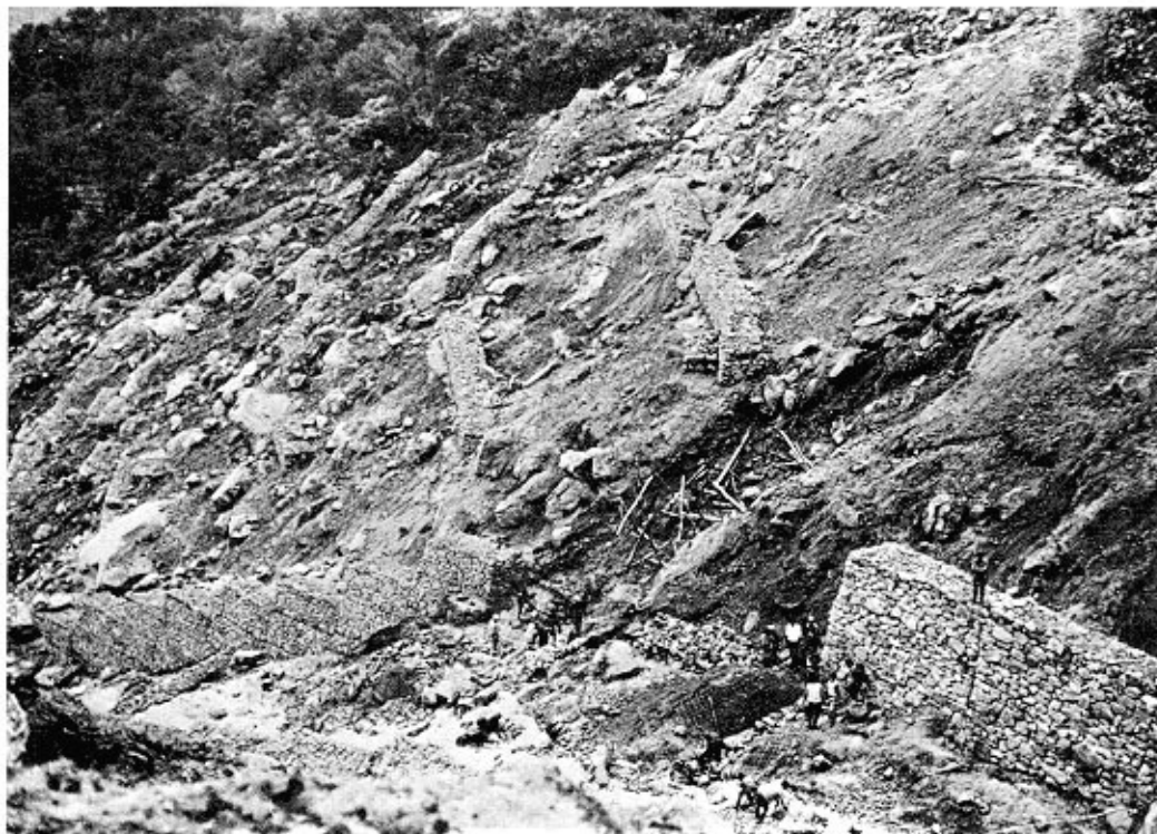
Fig. 15 Stabilizing steep hill slopes with series of 'sausage' wire-crated boulder retaining walls in the Teesta catchment (Sikkim) in the north-eastern Himalayan region
