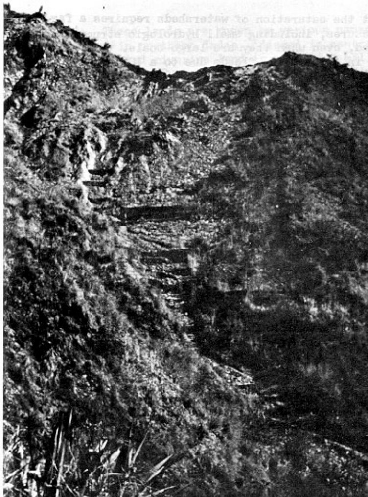
Fig. 14 Stabilizing torrents on hill slopes subject to landslides by a series of log and wire-crated (gabion) checkdams, mulching and afforestation at Dehra Dun, northern Himalayan region
