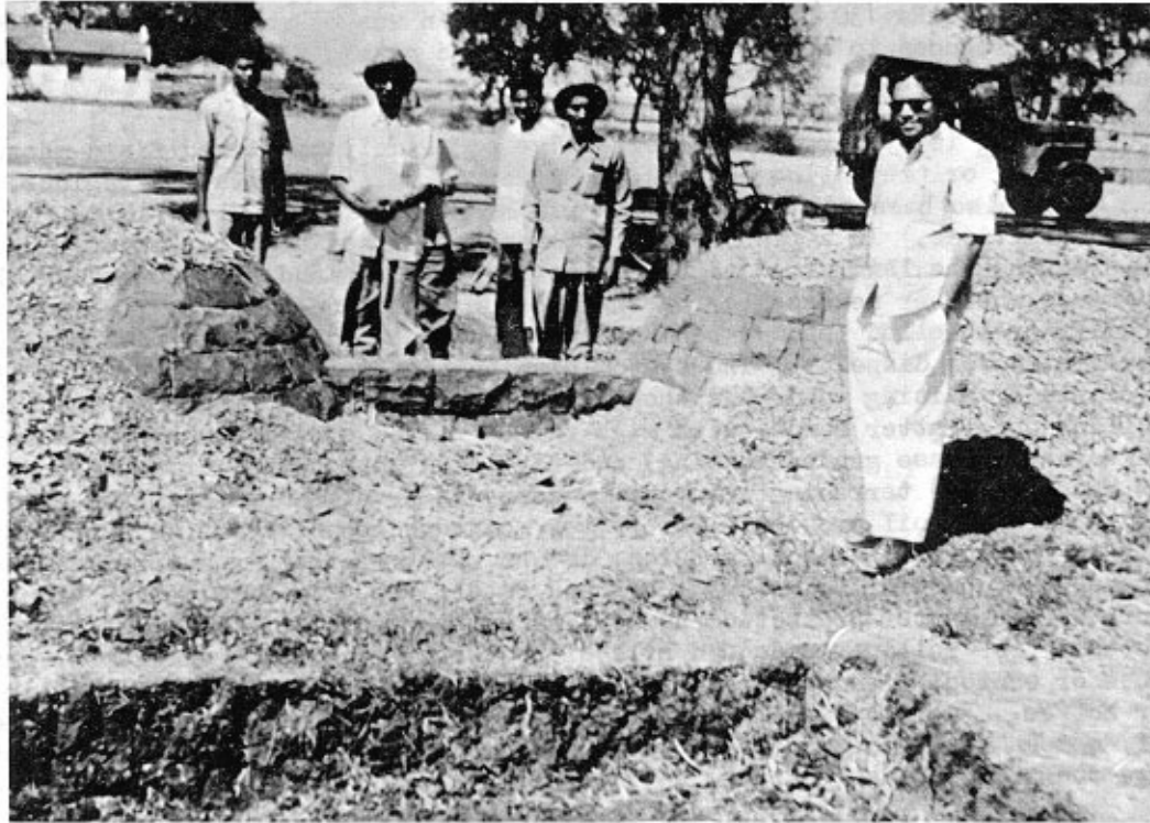
Fig. 6 Contour bunding (narrow base terrace on contour) with dressed rubble wasteweirs, in black soil region (shallow black soil)
