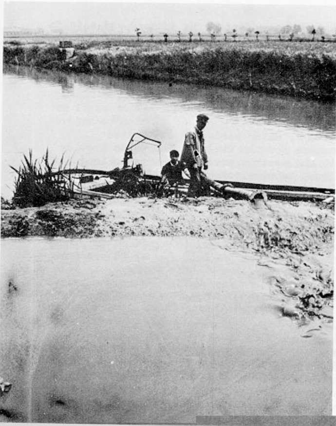
Fig. 6 Boat for sucking silt from the bottom of the canal. Foreground: Silt tank. Malu People's Commune, Shanghai
