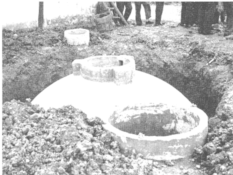
Plate 23. The biogas unit shown under construction in Plates 21 and 22, after its initial plastering. The outlet is in the foreground and the inlet in the background.
