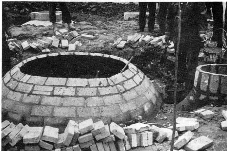
Plate 21. Constructing the dome of a biogas unit from bricks and using bamboo sticks to maintain the correct shape and angle. Note the nail through the stick for supporting the brick while cementing and, at the upper right hand side, the wire clamps temporarily supporting recently laid bricks. The outlet of the unit is on the extreme right. (Evergreen People's Commune, Hangzhou).
