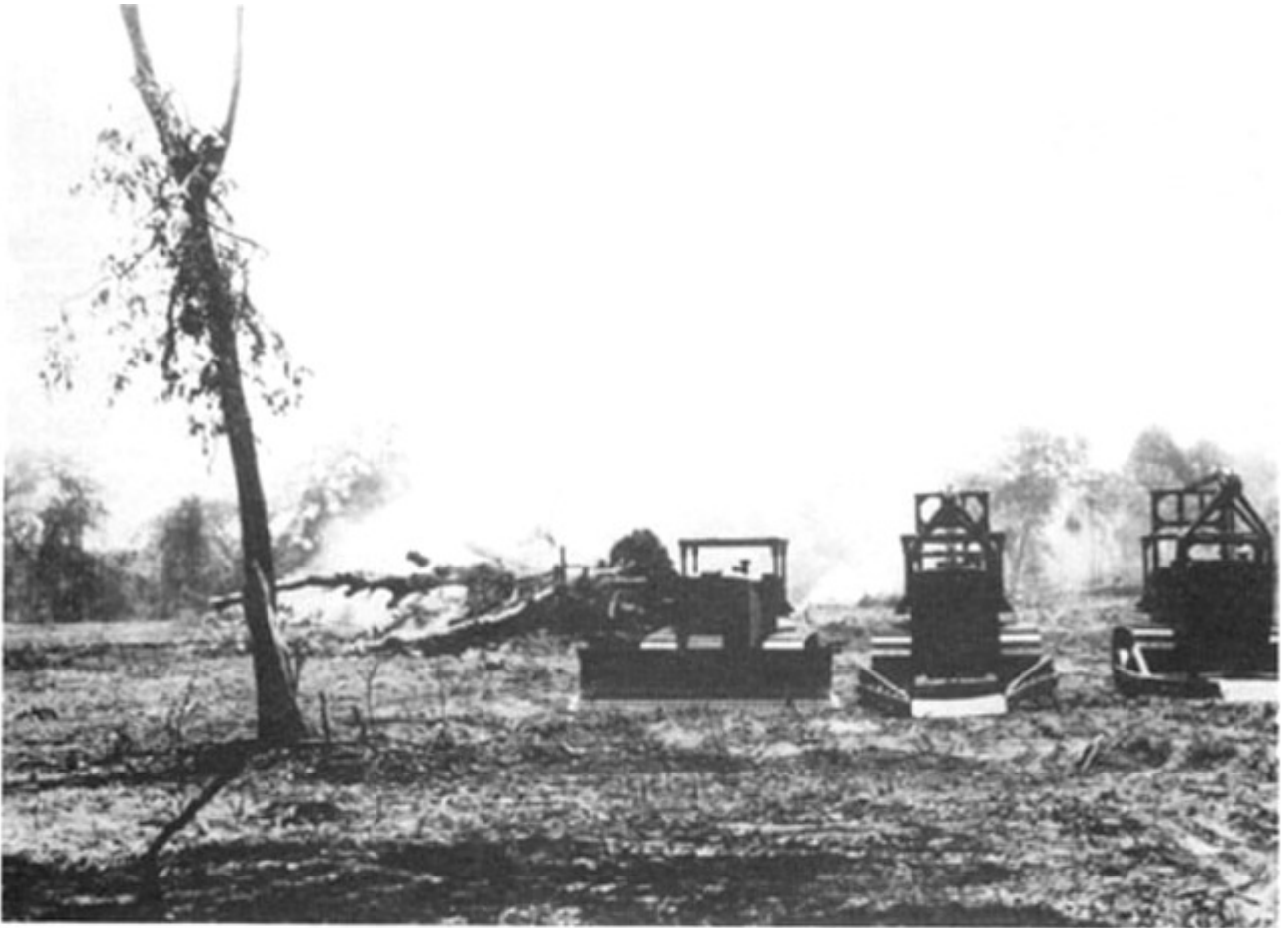
Fig. 46 Equipment used for jungle clearing in the Gal Oya valley of Sri Lanka. Heavy equipment may cause severe soil compaction, thus low water infiltration (FAO photo)
