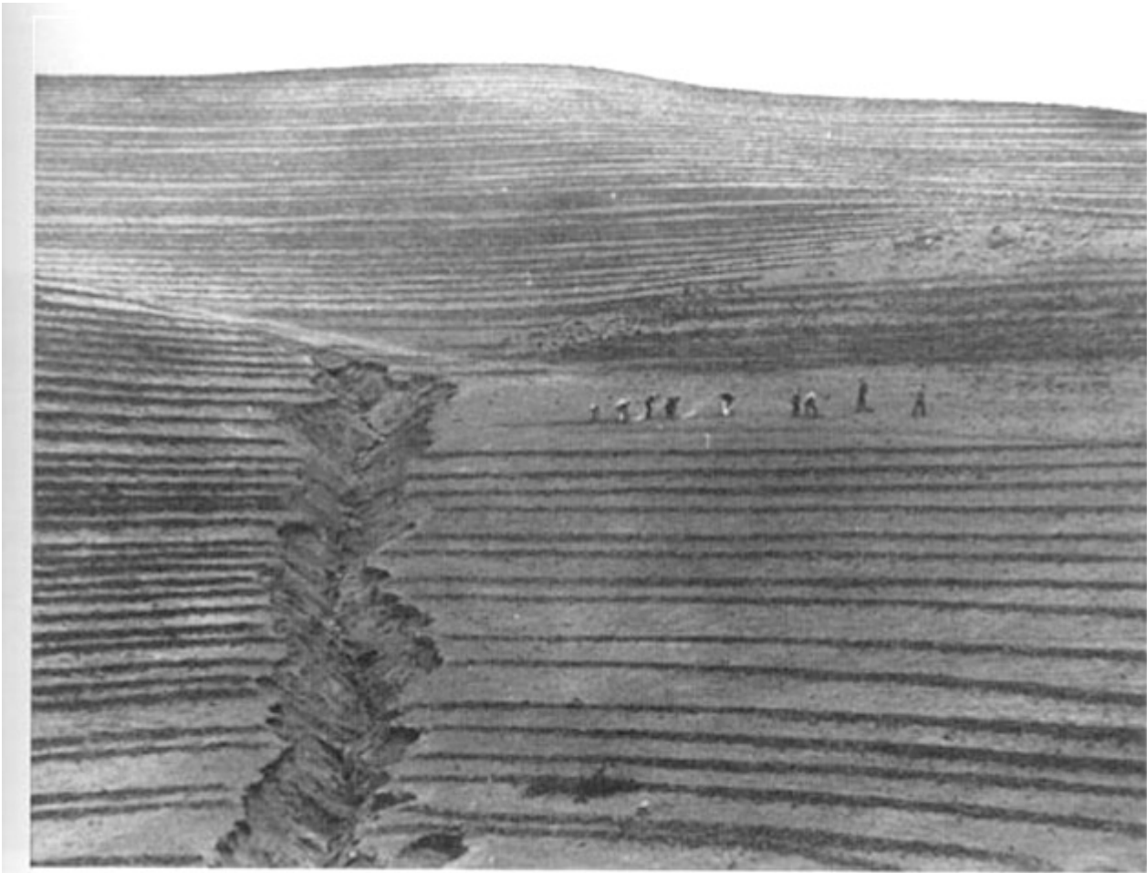
Fig. 59 Workers constructing ridges on the contour to help control erosion in Chile (UN photo, issued by FAO)
