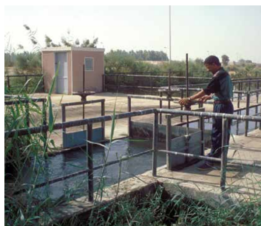
FIGURE 9.1 Water management plant and sewage water treatment station that filters underground and treated sewage water.
