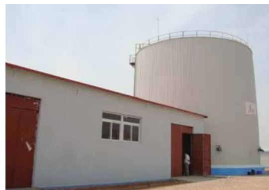
FIGURE 6.16 Biogas fermentation and biogas capture tank using straw fermentation on an industrial scale in Jinghai, Tianjin.
