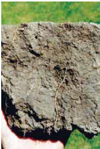
POOR CONDITION VS = 0 Soil colour has become significantly paler compared with under the fenceline.
